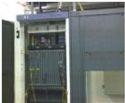
Shah Alam GPON project
